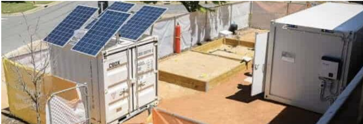
Testing site for hydrogen supplement in gas network - Canberra, Australia
