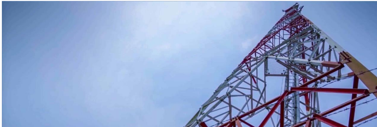
Telecom base station - Rompin, Pahang, Malaysia
